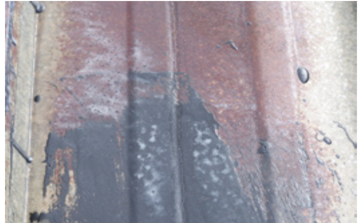
A section of the roof at Castle Hill RSL before it was treated with SkyCool.
