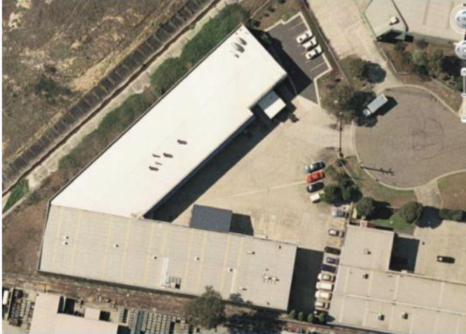
SkyCool's application to the roof of the South Western Sydney Area Health Service's food division, lengthened its life.
